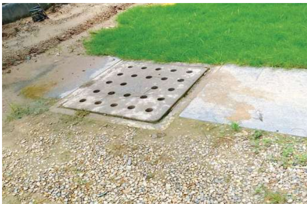
Storm water connection outside building premises
