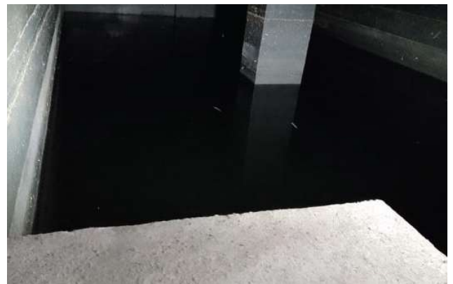
Rainwater tank at Basement 3
