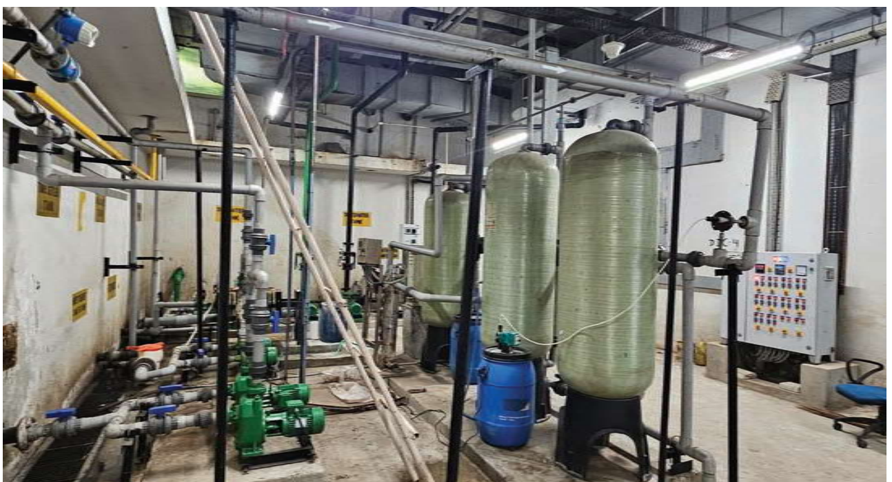
Sewage Treatment Plant (STP)
